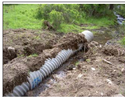
PHOTO #3: Winter wash-out of 2 nd Notch Road culvert shortly after installation in fall of 2007.
