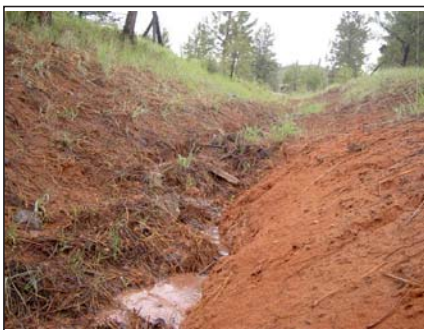
PHOTO #1: Eroded logging road before being "legalized" in 2007 by Wheeler County as a county road.
